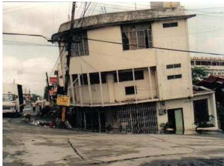
Figure 3-16: Tilted Structure after the 1990 Luzon Earthquake in Japan (Orense, 2011).
